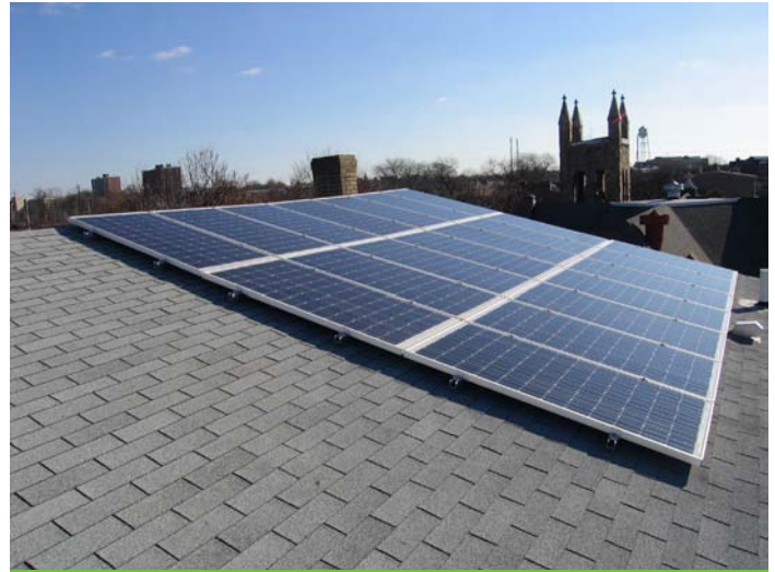
Roof-top solar panels
