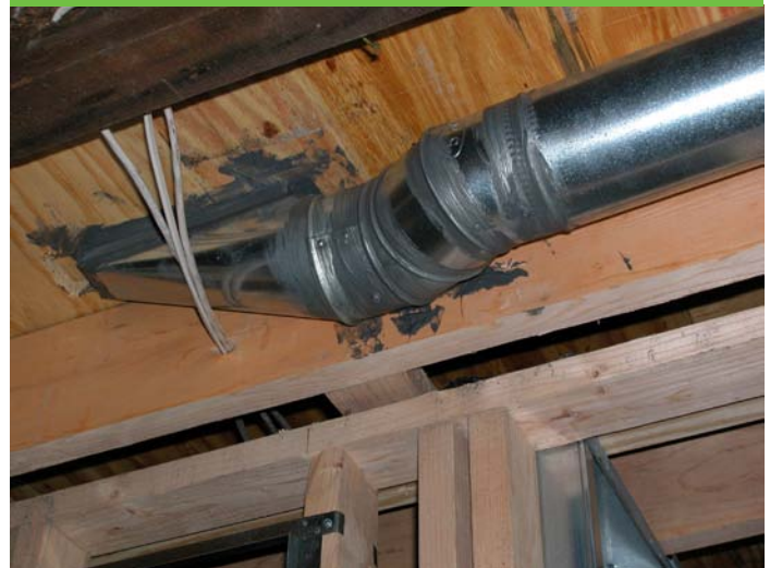
Ducts sealed with mastic
