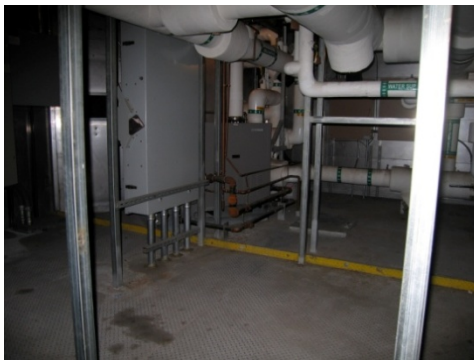
Fig 24: Mechanical room on ground floor Source: Clinton Andrews
