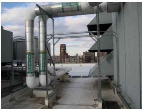
Fig 26: Mechanical systems mounted on roof area Source: Clinton Andrews
