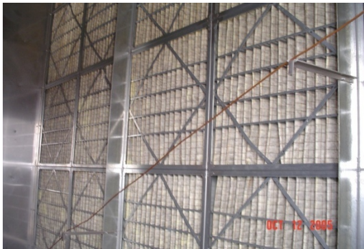
Fig 28: Filter media return plenum Source: Steven Martorana, NJEDA
