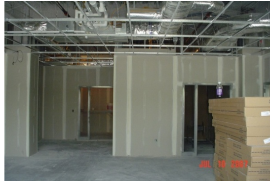
Fig 18: Floors kept clean during construction using sweeping compound to minimize dust Source: Steven Martorana, NJEDA
