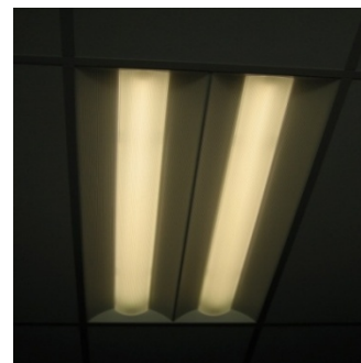
Fig 33: Energy efficient T5 fluorescent lights. Source: Clinton Andrews
