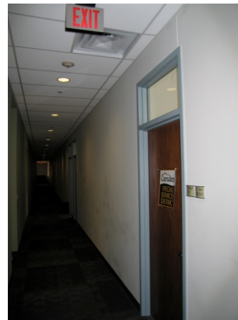
Fig 35: Compact fluorescent lights (CFLs) in corridors; Source: Clinton Andrews
