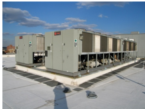
Fig 25: Air-cooled chillers Source: Clinton Andrews
