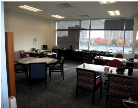
Fig 34: 46” T5 linear fluorescent lights in office areas; Source: Clinton Andrews
