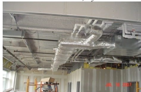
Fig 16: Protected ductwork Source: Steven Martorana, NJEDA
