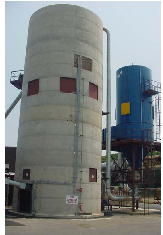
Biomass boiler (fuel storage silo is shown) at Rex Lumber, Englishtown, NJ. 150 kW cogeneration facility
