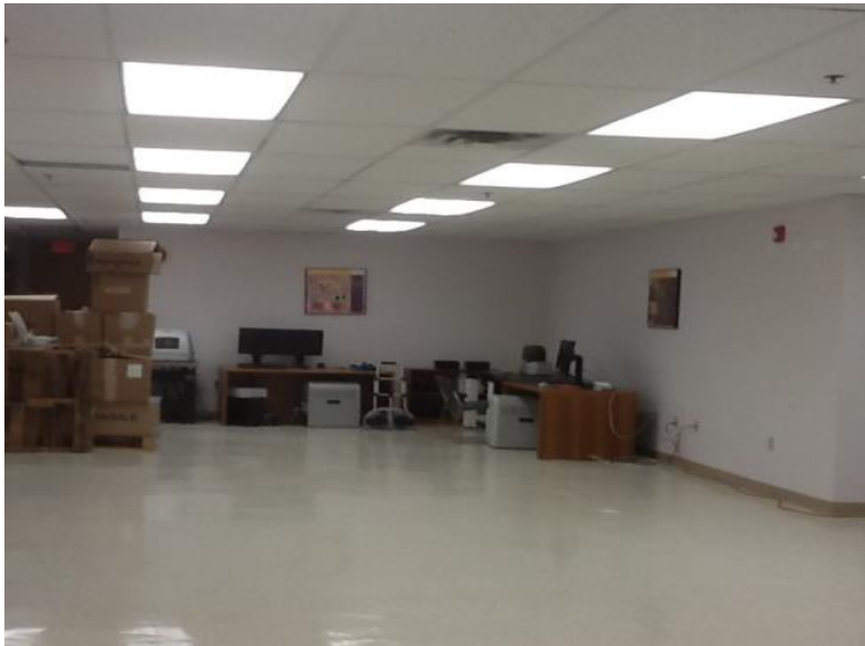
Inefficient lighting arrangement.
