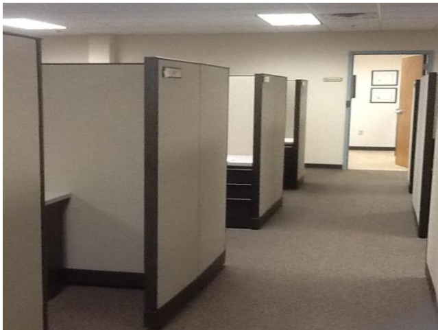
Misalignment of High Cubicles and Lighting Fixtures: ineffective from the standpoint of the user and may result in decreased satisfaction.
