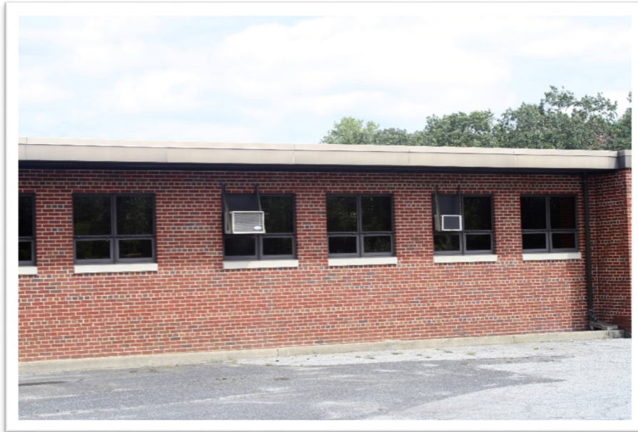
Photo: Window air conditioning units at the Hammonton National Guard site.
